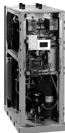
Access to control panel
