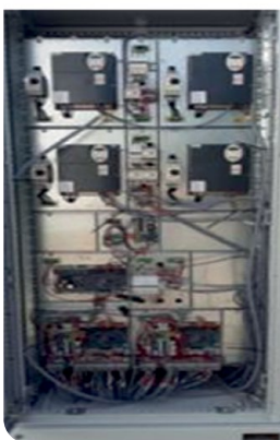
Fan drives + Pump drives + electronic boards
