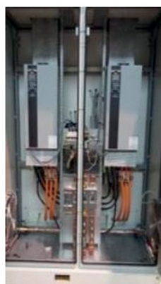
Compressor drives + main power connection
