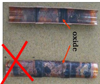
NO N2 to the pipes
